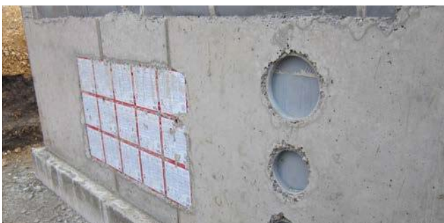
ZVR 150 and ZVR 200 set in concrete next to HSI 150
