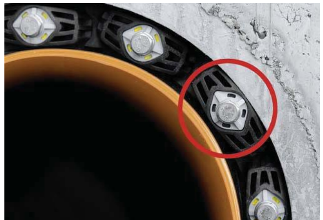
GKD with one segment not tightened – installation error immediately detected.
